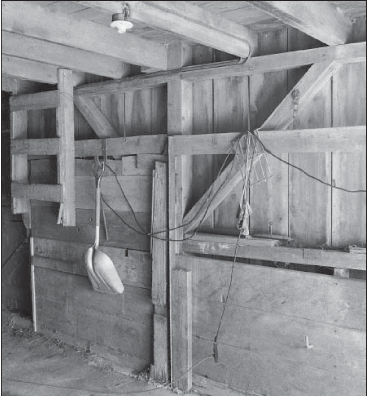
Ground level of the Howard barn with a scoop shovel and extension cords on the wall, 1994.
